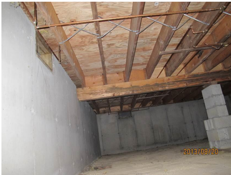
Viewing to left, front of left crawl space where two air vents are evident that should be closed
