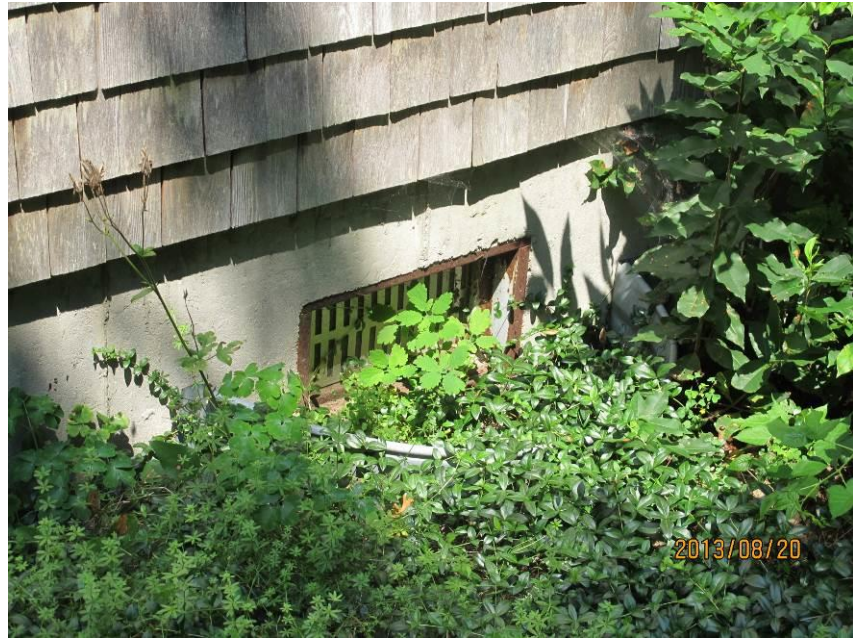
One of two air vents in to the right crawl space that was closed by Mr. Jones at the time of the inspection
