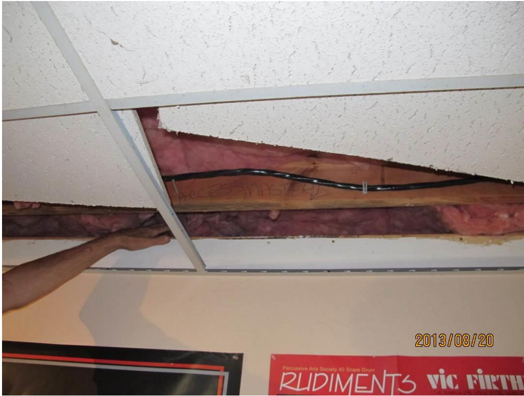
Fiberglass was pulled back to make MM reading of 18-19% MW in joist backing on left crawl space
