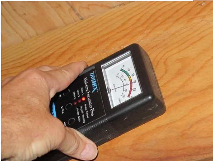
Unacceptable MM reading of 21+% MW in central joist
