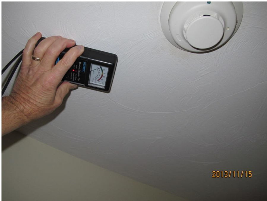
Dry MM reading in Beth's bedroom ceiling
