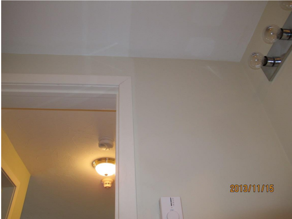
Area below leak in bathroom
