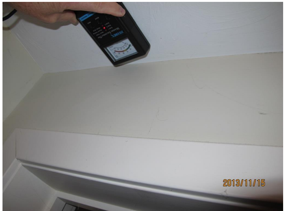
Dry MM reading in hall ceiling
