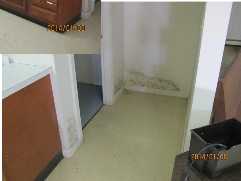
Cabinets on south side of “passage” backing on Ladies bathroom with VMG evident –suspect hidden mold growth as well
