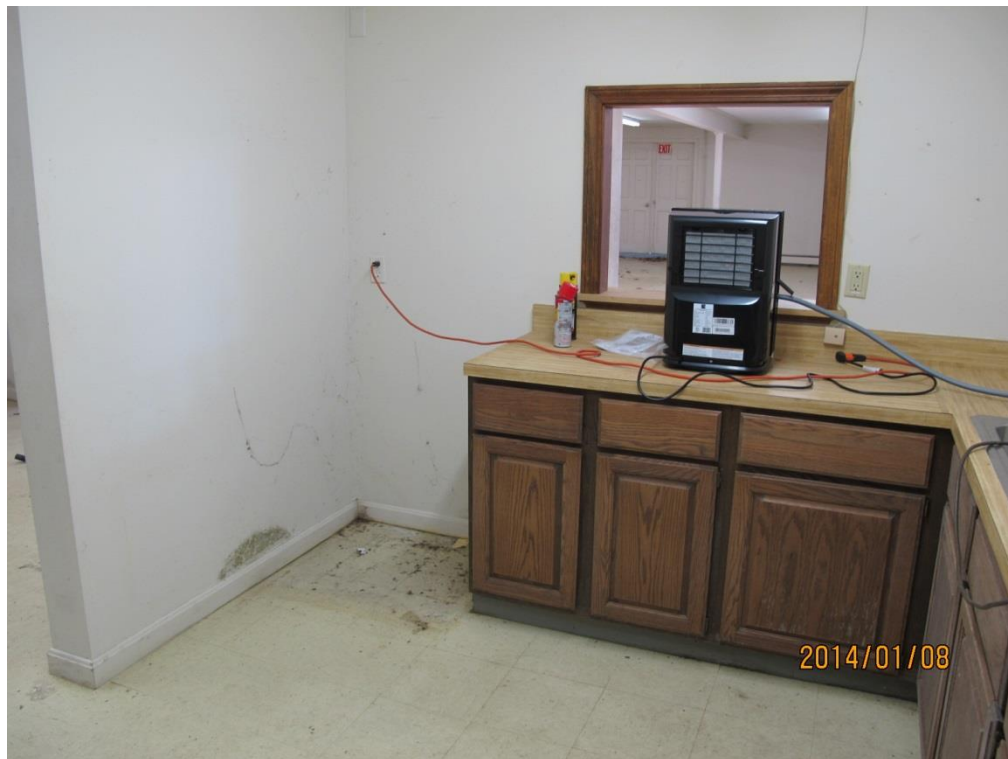
VMG near former refrigerator location, indicating possible leak
