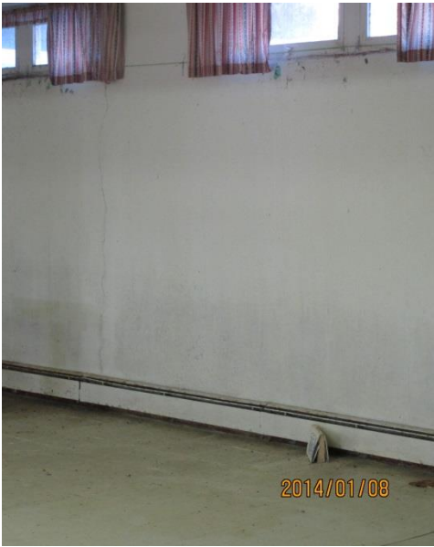
Haze of CMG along north wall
