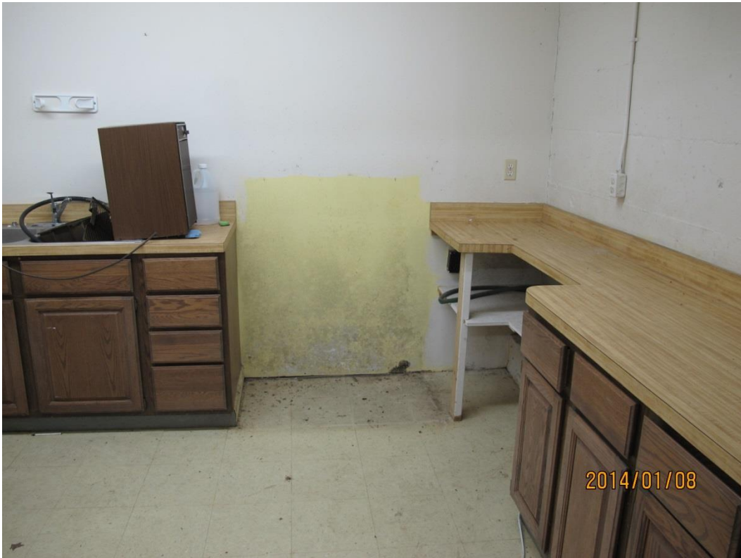
CMG on surface of wall behind former cabinet location with VMG near floor
