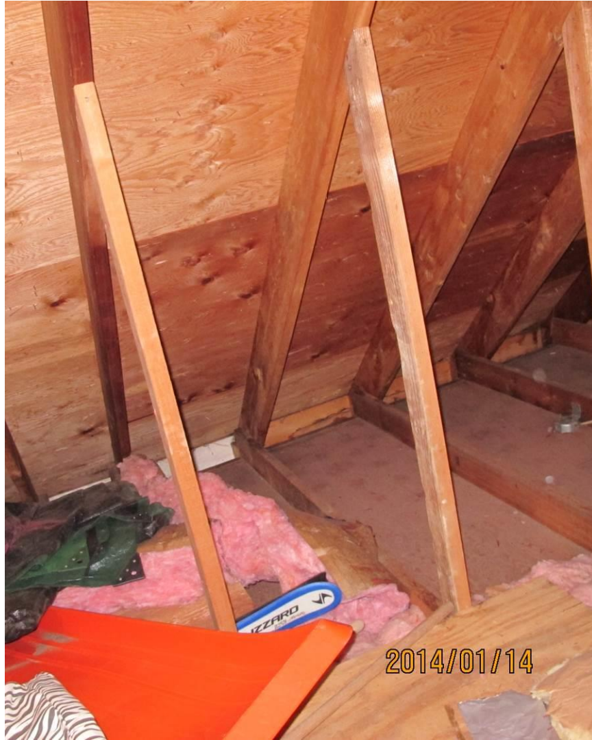
Front of garage room showing clear grain, nothing like the knee wall sheathing that was adjacent to occupied space where condensation on comparable surfaces supported in-grain mold growth
