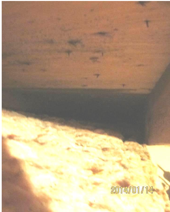
Straight line lumberyard mold growth indicating a sheet of plywood with different history from neighbors
