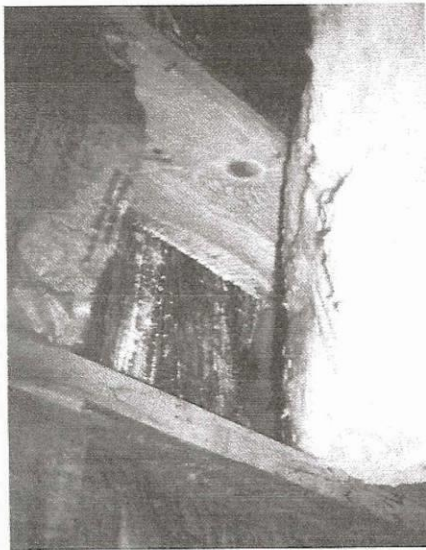
Rotted sheathing in a flat roof. The dark plywood sheathing between the lighter-colored rafters has been damaged by wood-decaying fungi. Water poured out of the fiberglass as the insulation was lowered, and the white semicircular threadlike pattern above the knot in the rafter is probably the mycelia of macrofungi that were starting to destroy the wood structure because of the saturated conditions.
