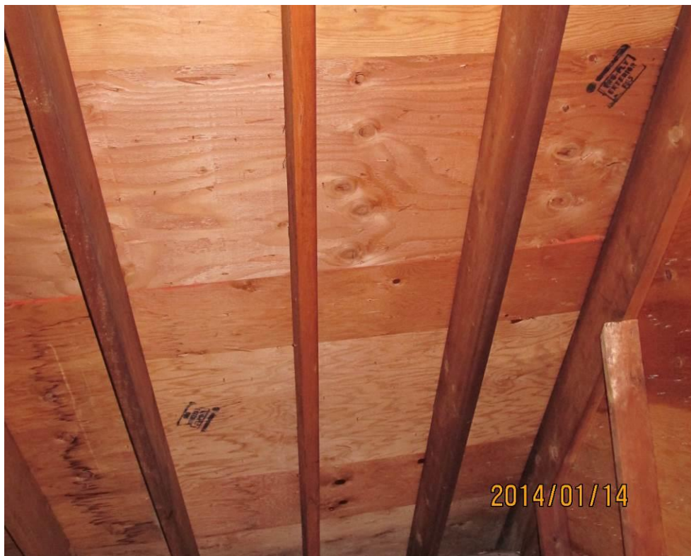
Right, rear of garage roof showing no signs of leaks that would have impacted garage ceiling
