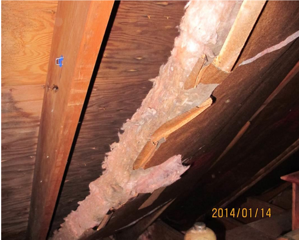
Gray material (dust/particle) at edge of insulation on left side
