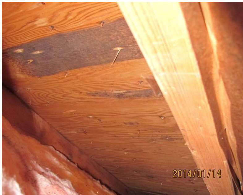
Isolated areas of condensation mold growth (lumberyard mold) in right knee wall area
