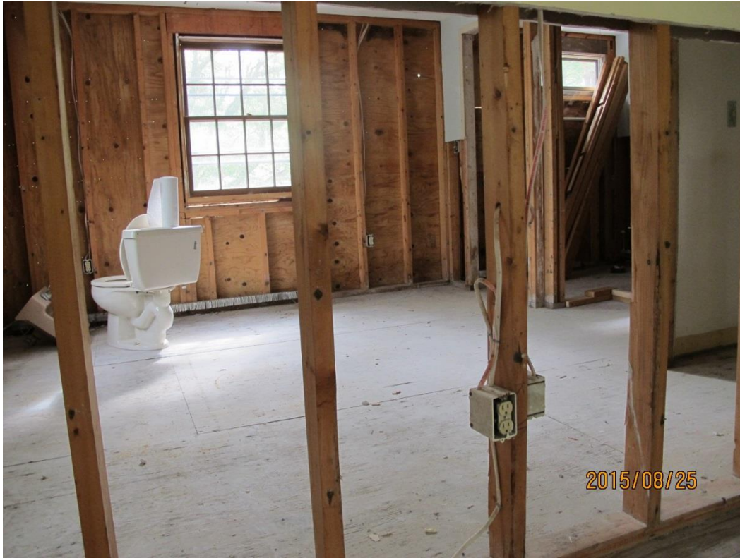
Left, rear bedroom off bathroom with leak
