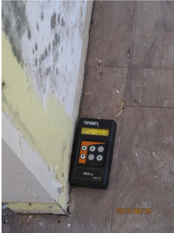
Sub floor in kitchen reading 22+% MC
