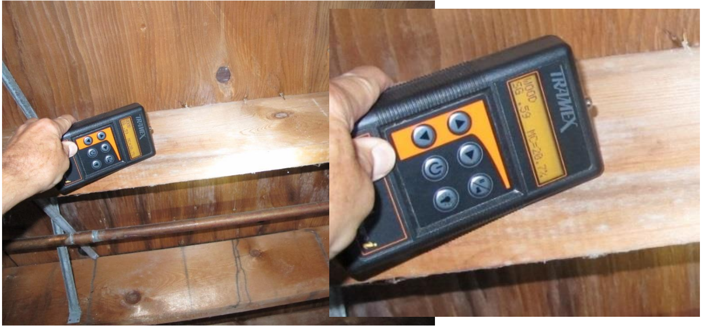
Unacceptable MM reading of 20.y% MC in joist
