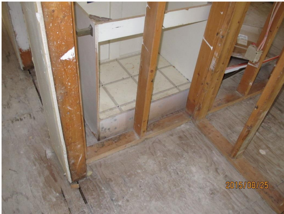
VMG on rear of vanity and on sill board
