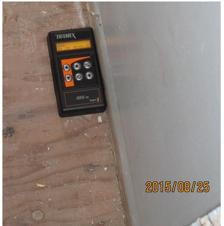
Subfloor in bathroom reading 24+ MC
