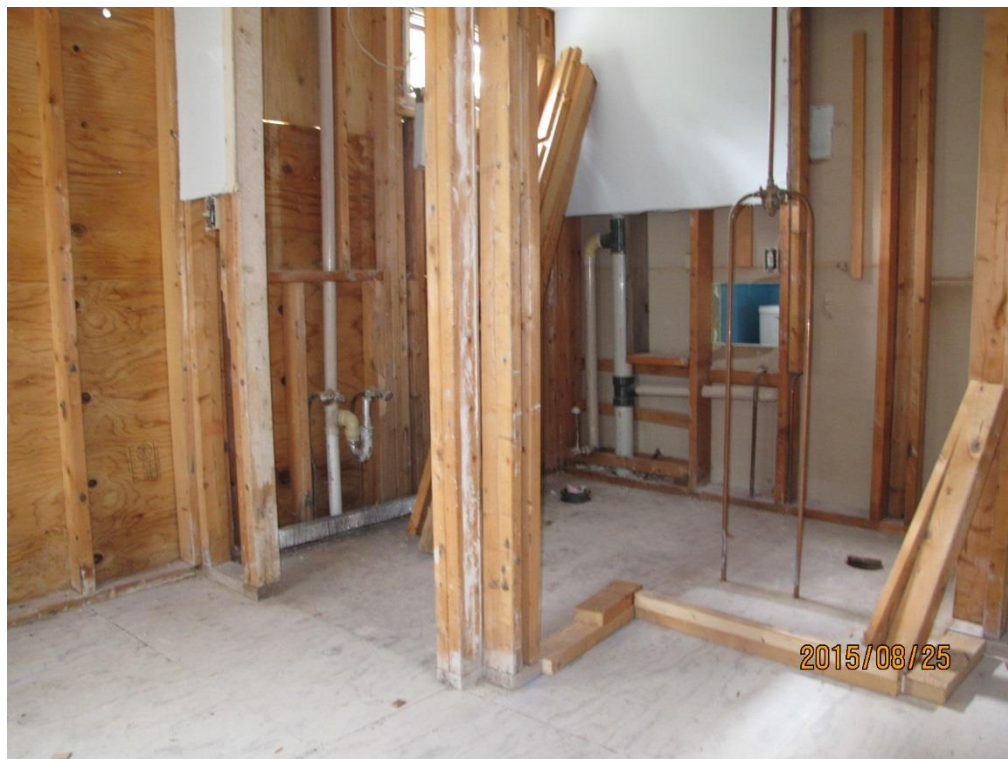
Bathroom where leak occurred at rear sink
