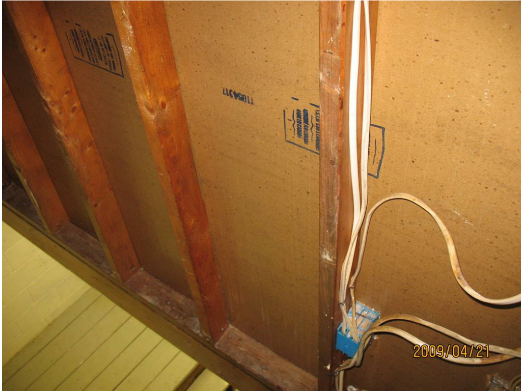
Absence of VMG on drywall going down basement steps
