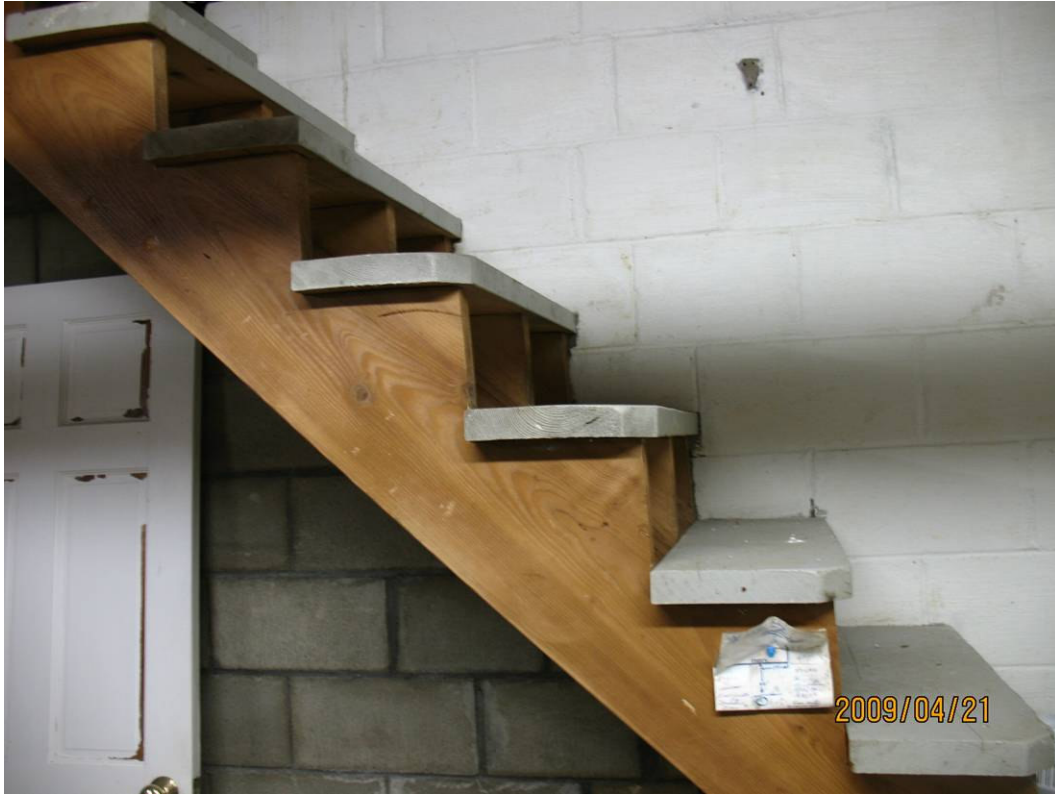
Absence of VMG on basement steps
