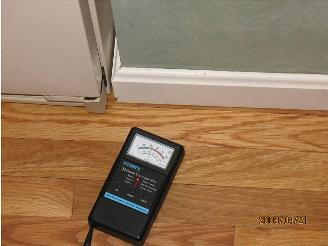
Satisfactory MM reading near the refrigerator
