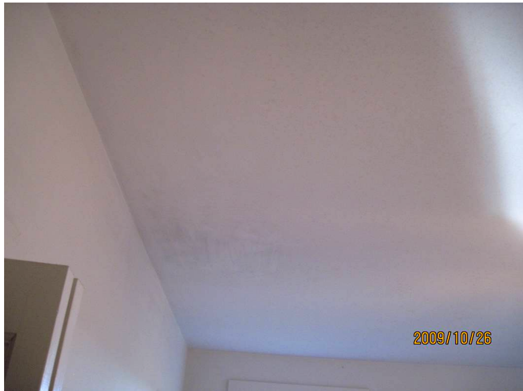
Blotchy CMG on left rear bedroom ceiling
