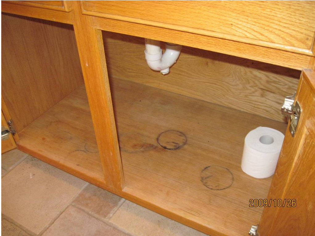
Rust stains under bathroom sink but no mold growth
