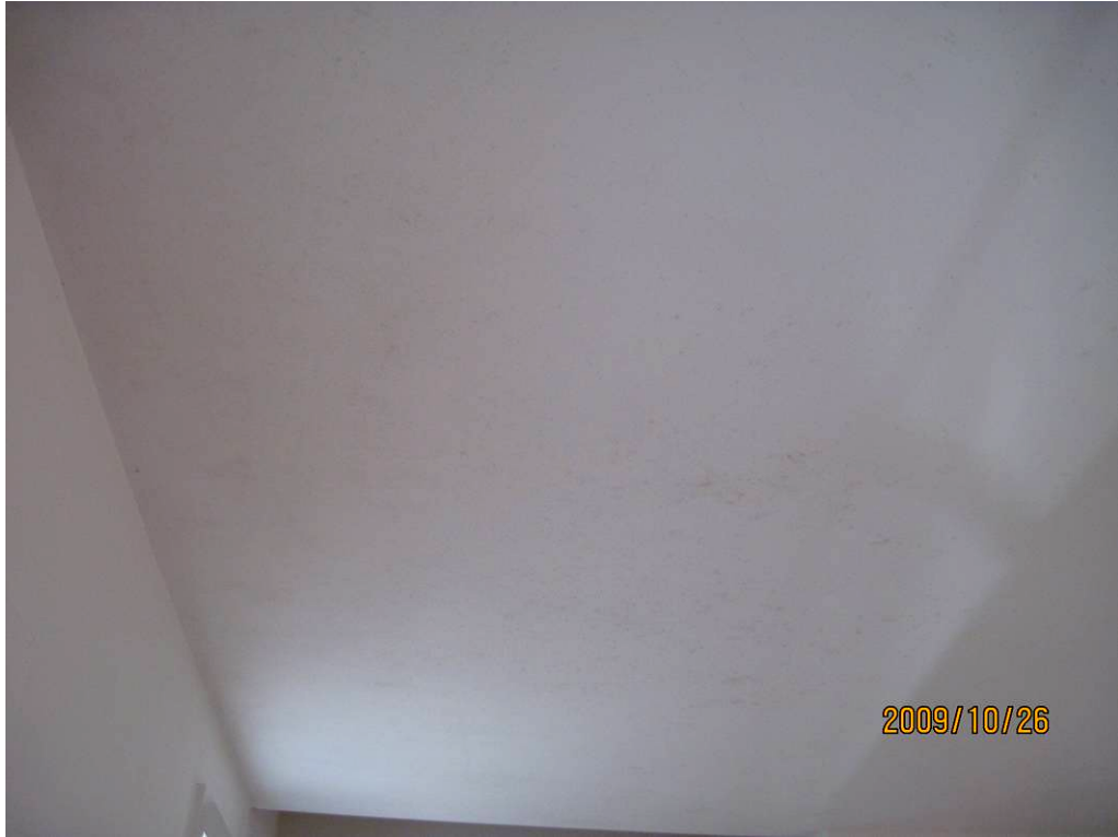
Blotchy CMG on living room ceiling
