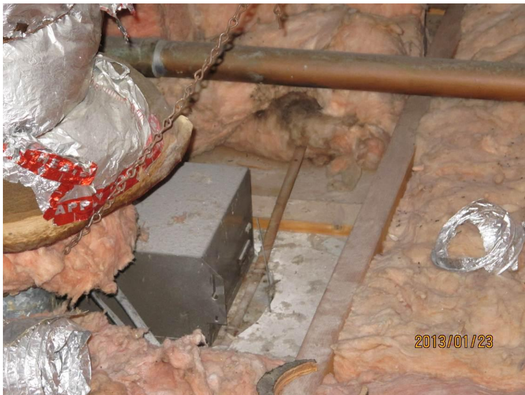
Area near bathroom exhaust fan showing large uninsulated surface (compare to earlier view of VMG)
