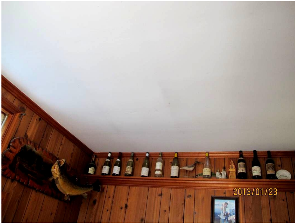
Hazing/ghosting in right rear paneled room
