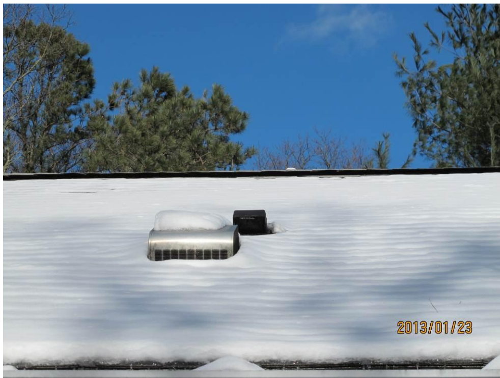
Vents from the bathroom area – large = shower & small = dryer
