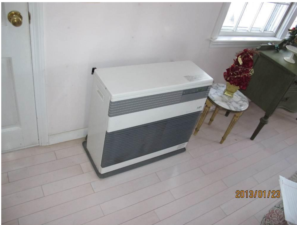
Monitor wall-mounted heater in living room
