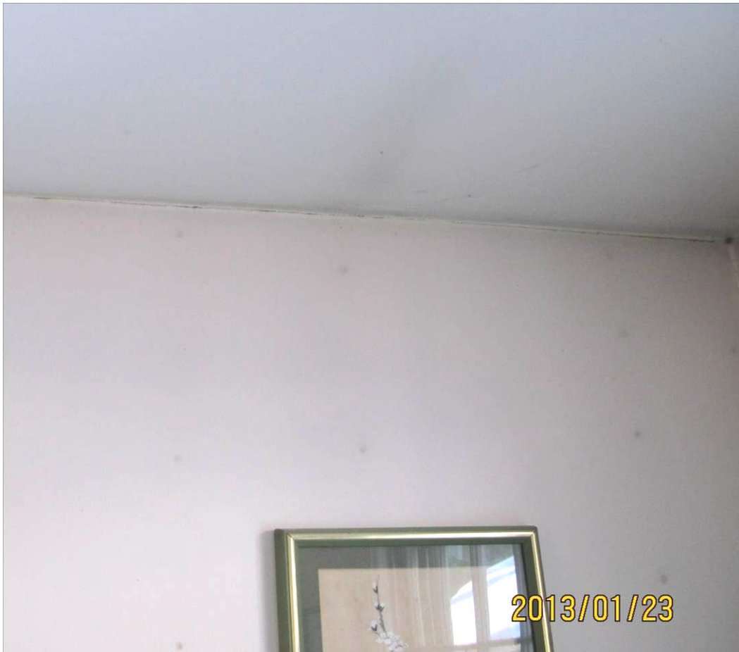
Drywall nails and ceiling corners showing hazing/ghosting on front wall
