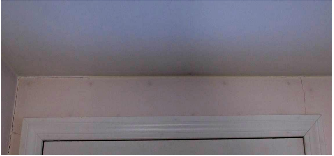
Drywall nails evident over front door
