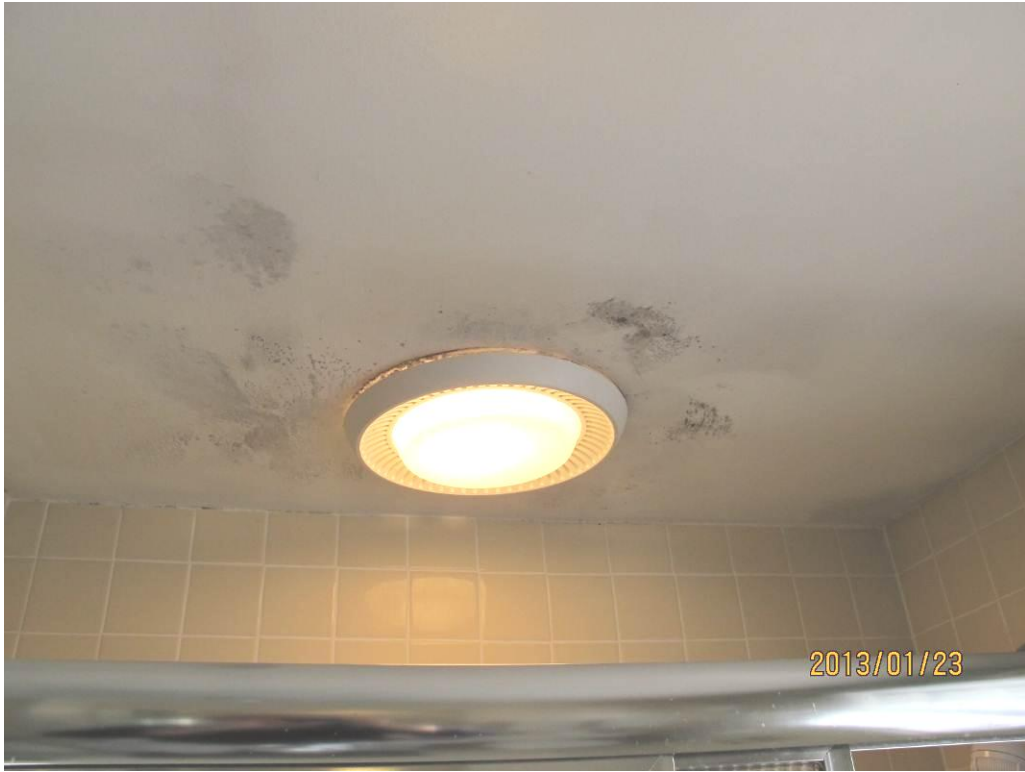
VMG around shower exhaust fan
