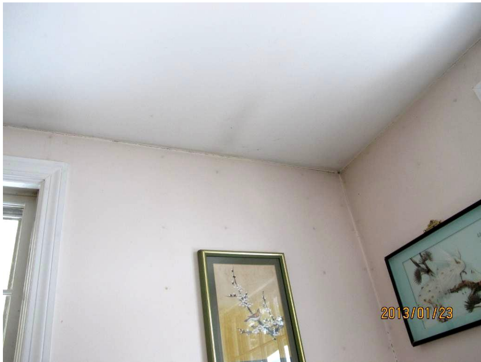
Hazing/ghosting along front wall and right corner of living room
