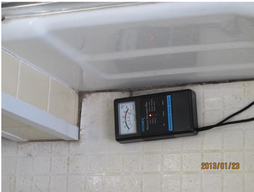
Excess moisture (28% MW) in bathroom floor near foot of tub/shower
