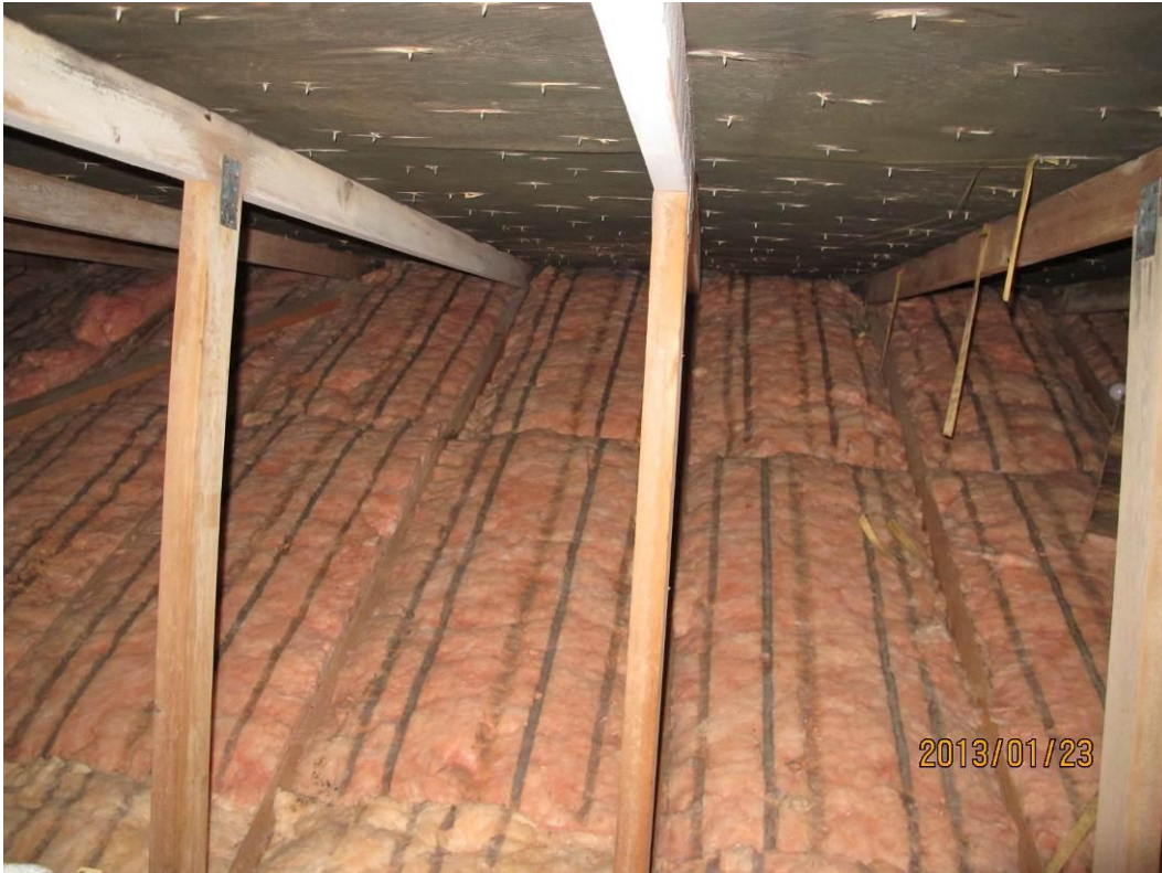
Insulation on north side of attic where there is an evident dip in the insulation where batts are not fully butted together, leading to cooler, linear surfaces in the ceiling below
