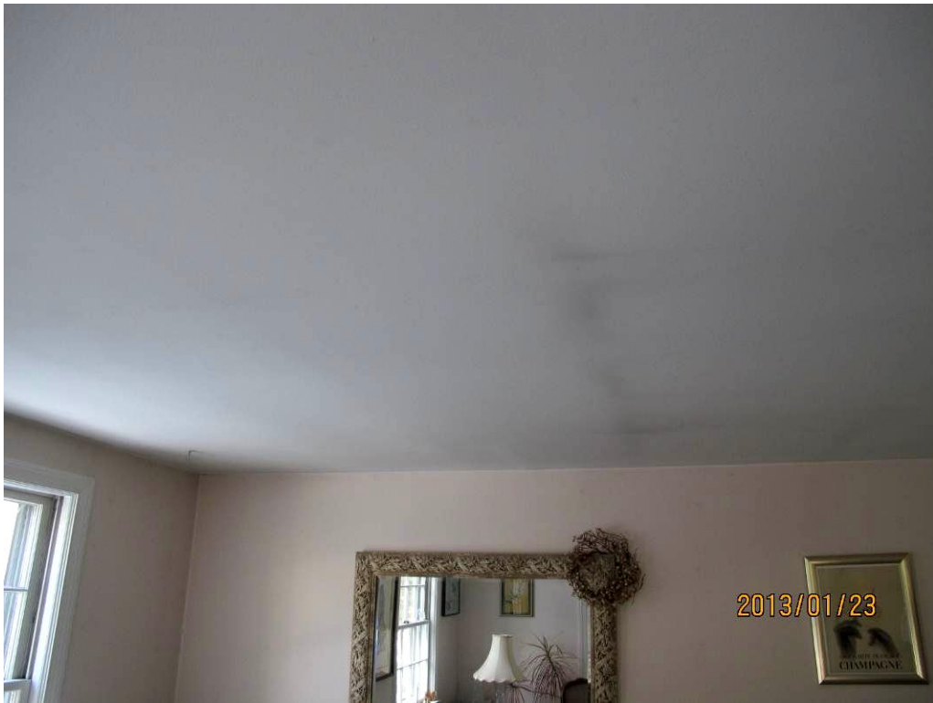
Hazing/ghosting on living room ceiling (see attic discussion & photos as well)
