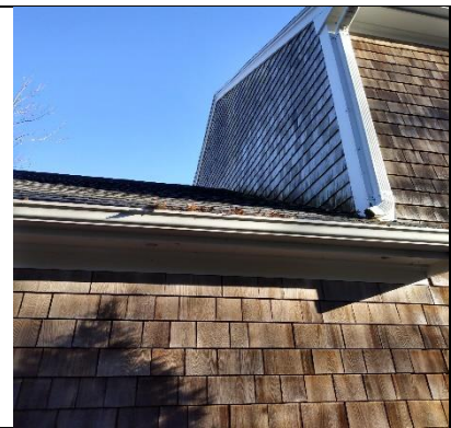
Note debris in the gutter. Also note the small, "hockey puck" style soffit vents that extend around the house which may contribute to inadequate attic ventilation.
