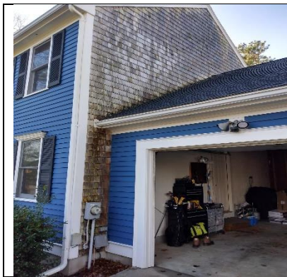
Note how wet the cedar shingles on the north-facing gable end, particularly the section immediately opposite the attic.
