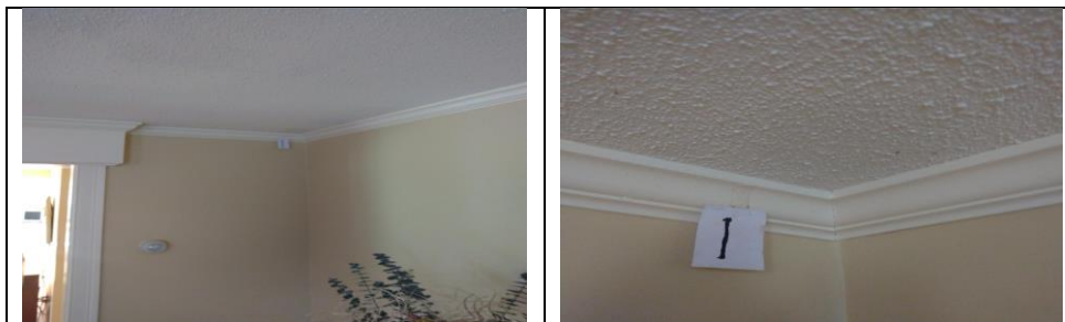
Living Room Ceiling – distance view to left and close-up to the right
